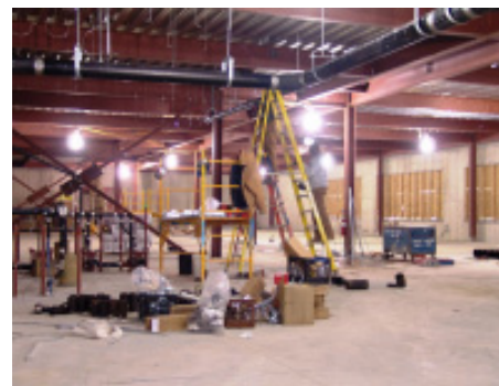
The building is totally enclosed and work is underway on the 70,000-square foot interior
